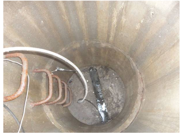
Picture#89: Central manhole to be repaired (1.4.4)
