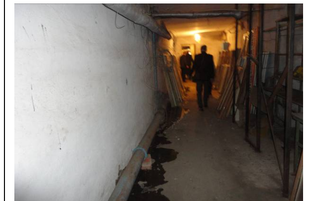
Picture#85: Leaking piping to be replaced or repaired along the basement hallway (1.4.2)
