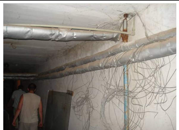
Picture#93: All sewer connection piping in the basement of the West Wing to be replaced (1.4.1)
