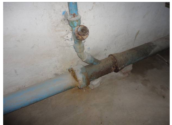
Picture#91: Leaking piping to be replaced or repaired along the basement hallway (1.4.2)
