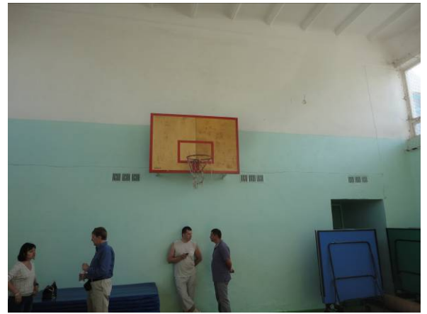
Picture#59: Basketball board and ventilation wall louvers to be replaced
