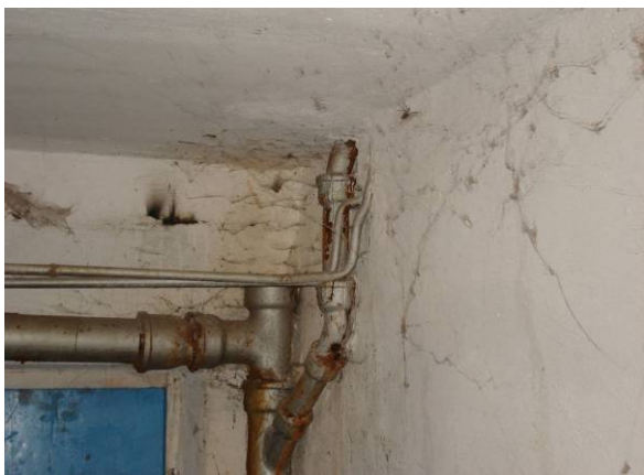
Picture#84: Sewer piping to be replaced (1.4.1)
