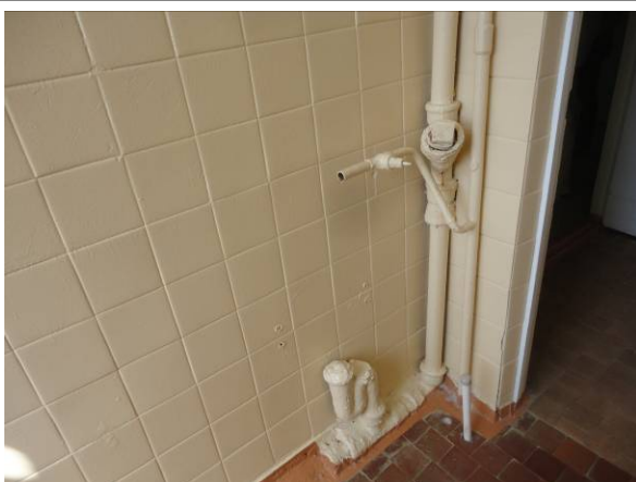
Picture#38: All piping to be removed and replaced with new to be recessed within the new wall surfaces.
