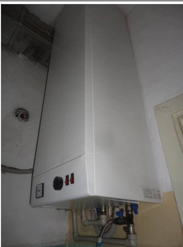
Picture#70: Existing water heater to be reutilized and supplemented with a new one.
