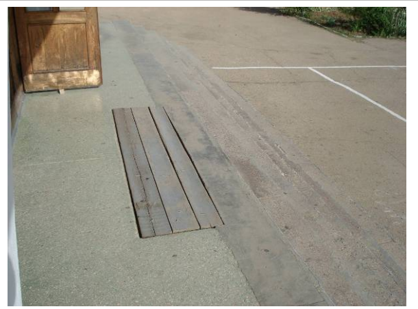
Picture#106: Existing space that used to be used to clean shoes. Landing platform to be new at the same height as the existing.
