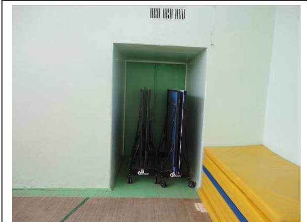
Picture#56: Door to be replaced.
