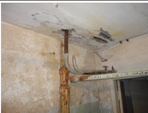
Picture#86: Sewer piping to be replaced (1.4.1)
