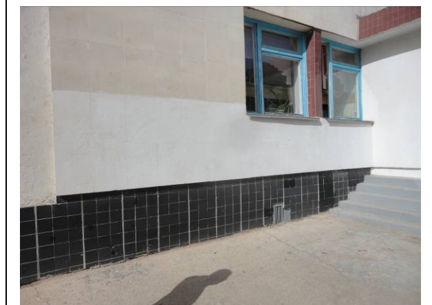
Picture#96: Remove all ceramic tiles. The lower part of the natural stone tiles is painted. Paint to be removed.
