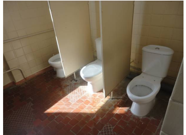
Picture#35: Typical girls' toilets in West Wing. All to be replaced with new.
