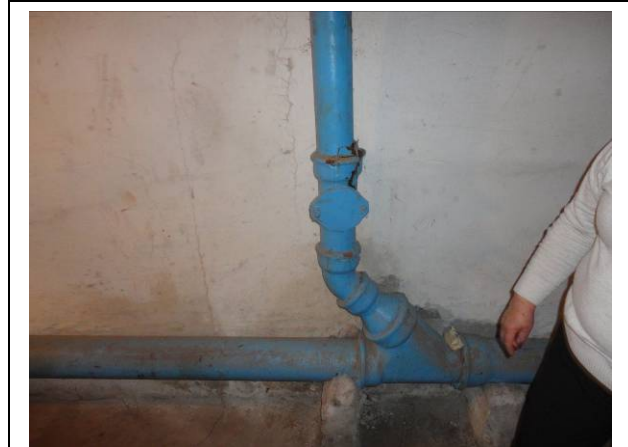
Picture#87: Connection from sewer piping to be replaced (1.4.1) to main sewer line to be repaired or replaced (1.4.2)
