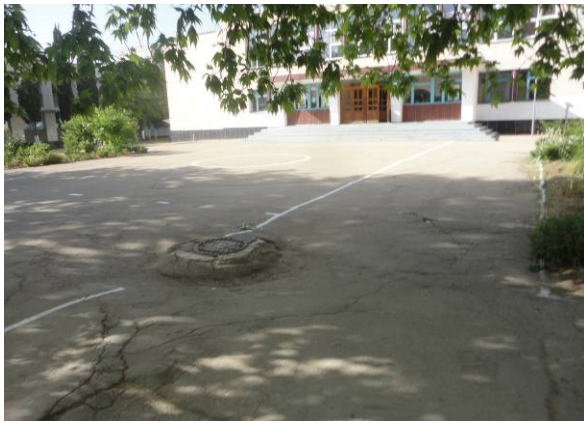
Picture#82: Central manhole to be repaired
