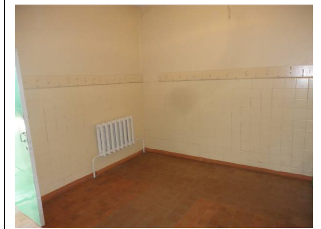
Picture#66: Interior of locker rooms. Replace radiators. Provide new ventilation to the exterior of the facility to avoid bad smell.
