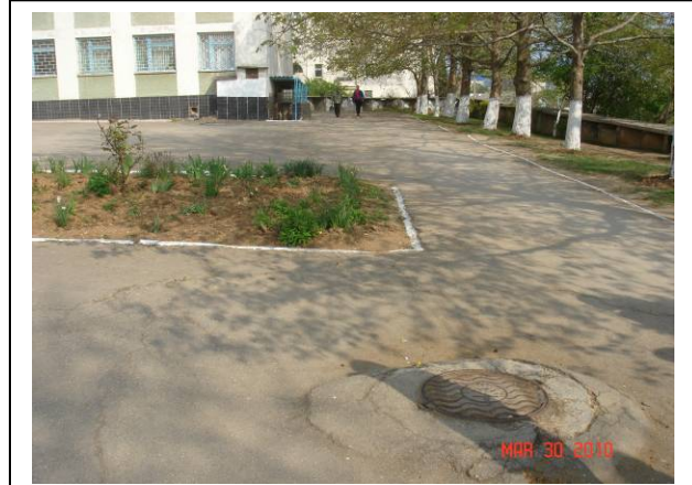
Picture#83: Central manhole to be repaired
