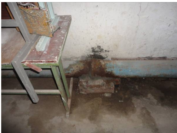
Picture#90: Sewer piping to be repaired or replaced (1.4.2)
