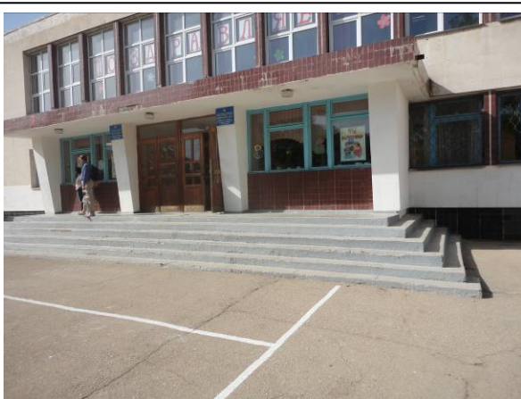
Picture#99: Steps to be repaired by replacement.
