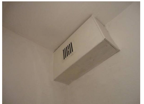
Picture#31: Replace ventilation system and put under new drop ceiling
