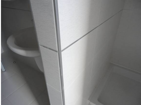
Picture#28: Typical aluminum with anodized finish corner protection. This is required in all corners of new ceramic tiles vertical walls.
