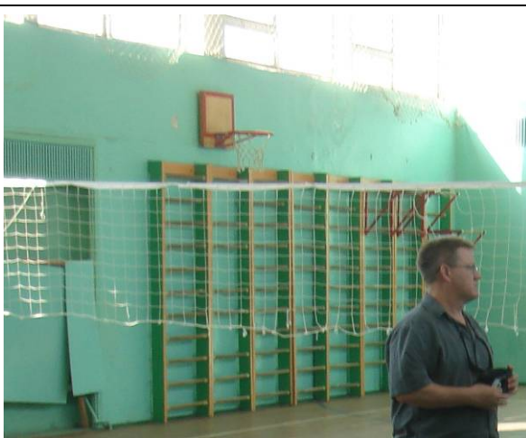
Picture#60: Existing wood racks and secondary basketball board to be replaced with new.
