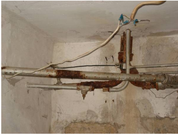
Picture#88: Typical lines to be replaced (1.4.1)
